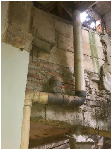
(a) Pipes water
