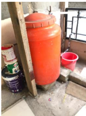
(a) Water tank
